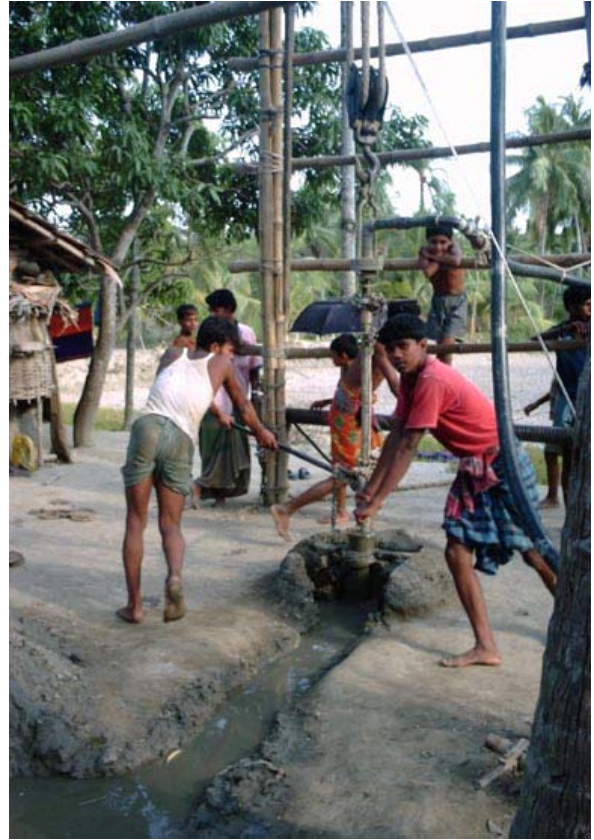
A DTW digging site. Two workers walk around continuously on shifts holding the levers attached to the drilling pipe day and night.
